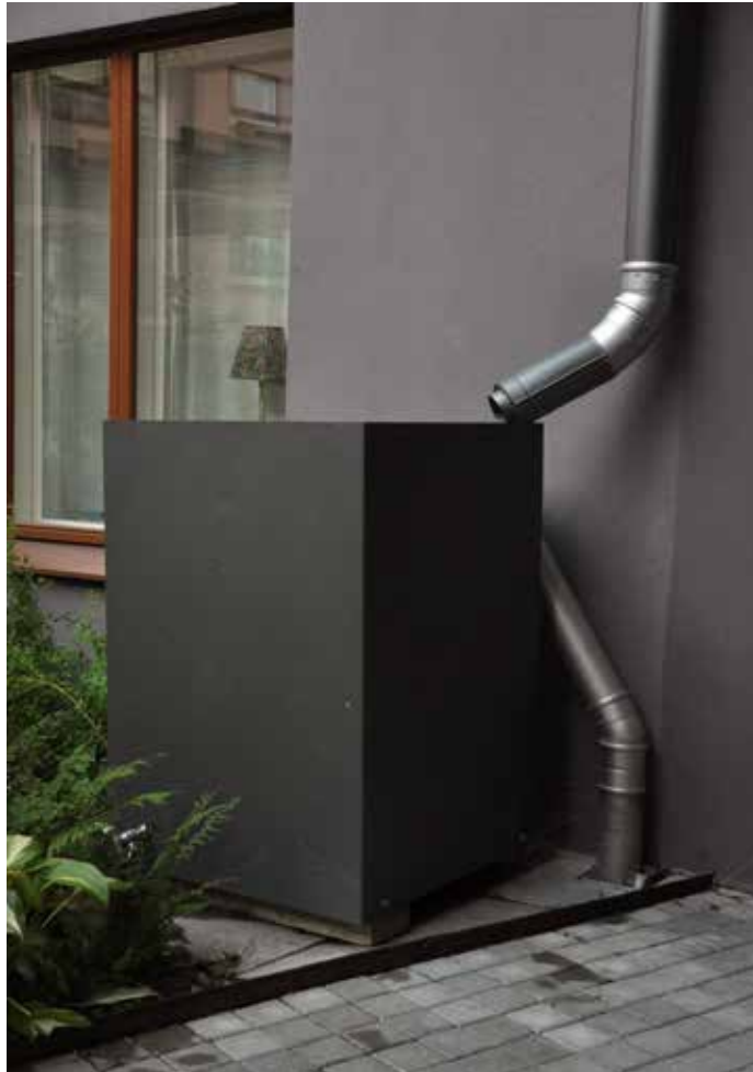
Figure 53: Examples of concealed tanks used for rainwater harvesting.
